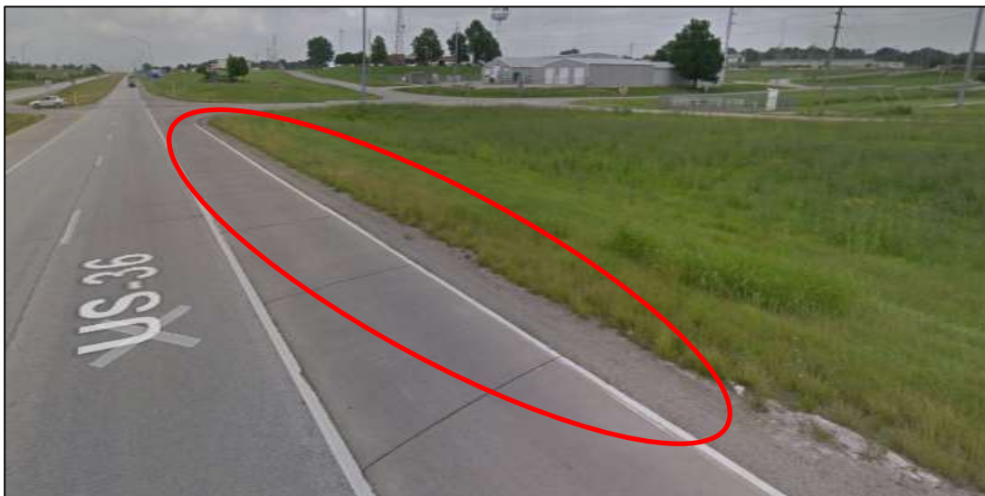
Figure 19 – Westbound US Highway 36 Shoulder
