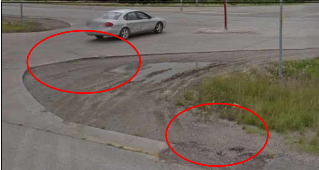
Figure 16 – Potholes and Drop Offs
